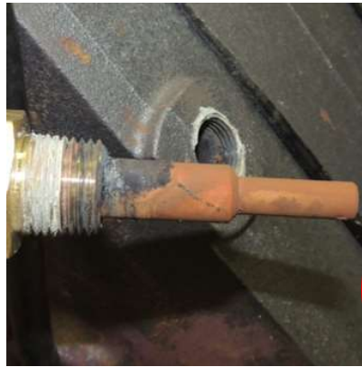
LWCO Probe fouled
